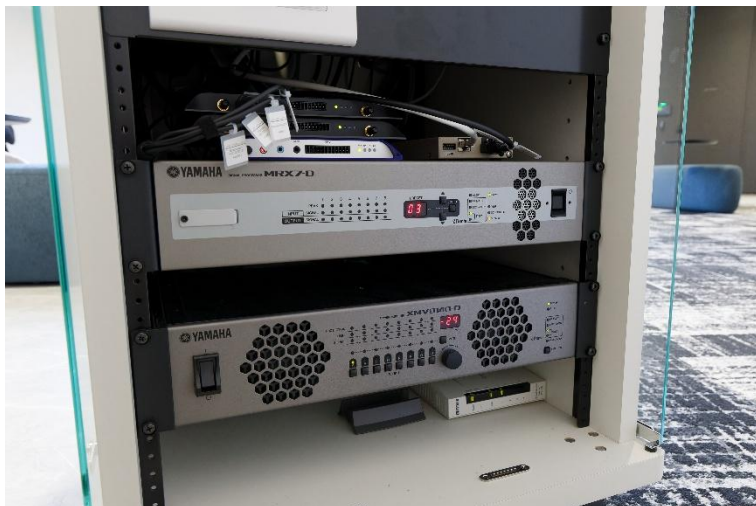
MRX7-D signal processor (top) and XMV8140-D power amplifier (bottom)
