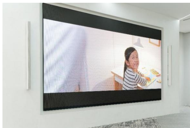
VXL1W-24 speakers installed at entrance signage
